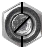
(Bolt is loose)
