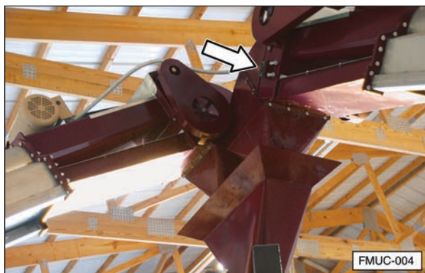
Conveyor Belt Upper Roller (both sides)
